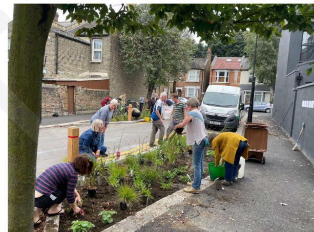
Figure 17-9 Community Rain Gardens project in Waltham Forest, UK - image © Meristem Design. Source: NTA, Greening and Nature-based SuDS for Active Travel Schemes Advice Note.
